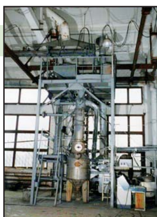
General view of the gasification installation created in Project 651
